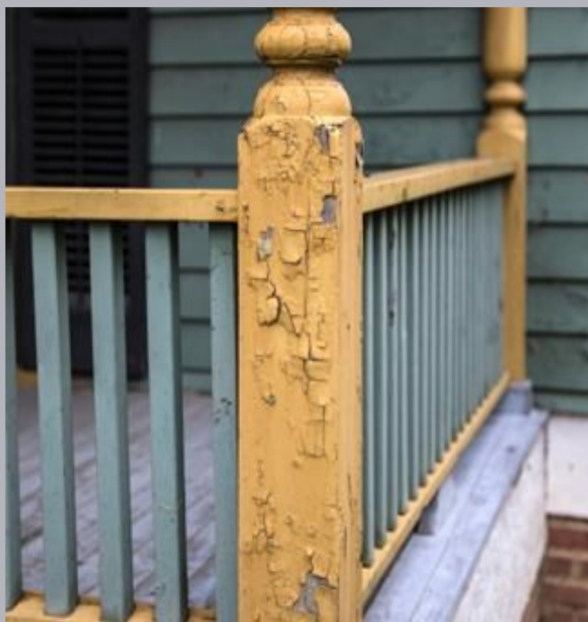
An example of lead paint on porches
