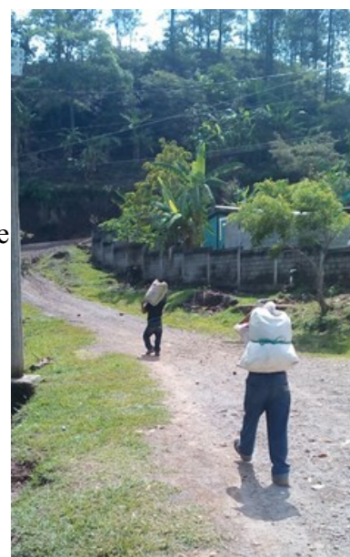
Beginning to carry 100 lb bags of cement up hillside. Each pila requires carrying 6 bags
