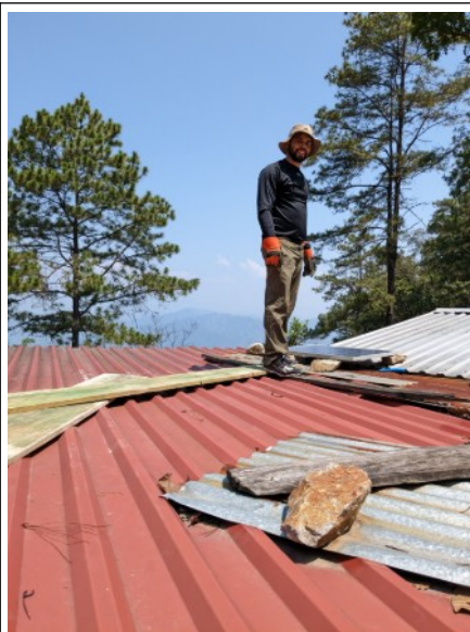
Yoni doing a great job installing a solar panel on a roof
