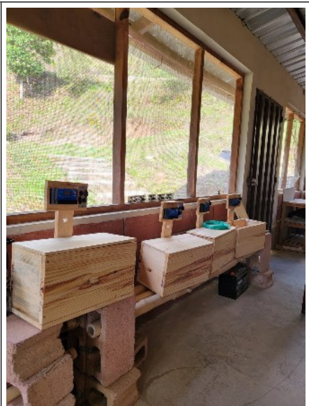
Locally made battery boxes wired up and ready for installs
